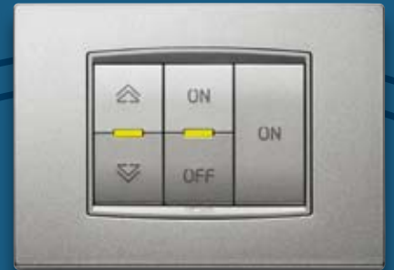
Lights and automations control. The groups of lights and groups of motorized blinds are controlled from here, for the greatest cruise comfort.
